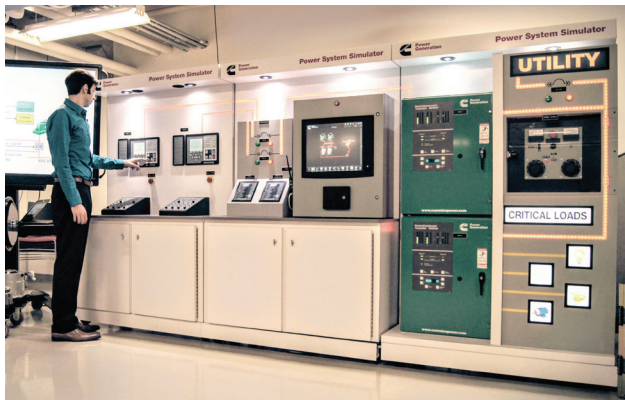
The Power System Simulator in the Cummins Power Generation Customer Experience Room.
