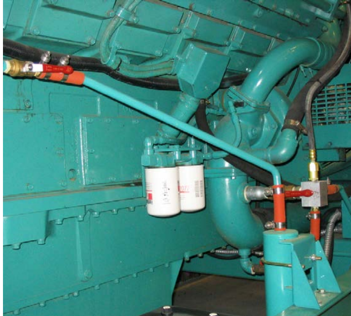
Temperature Maintenance and Cooling Systems
