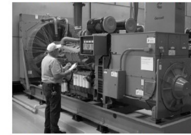
A well-planned maintenance program is essential to the operation of any power generation system.
