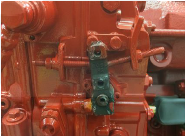
Figure 5-4 Fire pump drive engine threaded linkage rod
